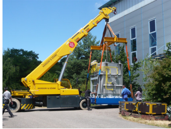
Fig. 3: VPC melter taken out of the technical hall of KIT-INE for transport to China
