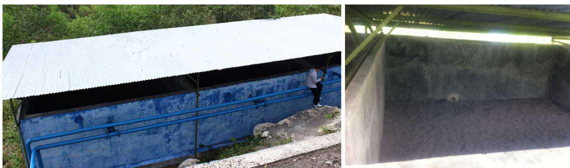
Fig. 6 Left Slow sand filter plant. Right One chamber filled with lava sand as filter material. Currently, on-site validation is being conducted by Indonesian project partners
