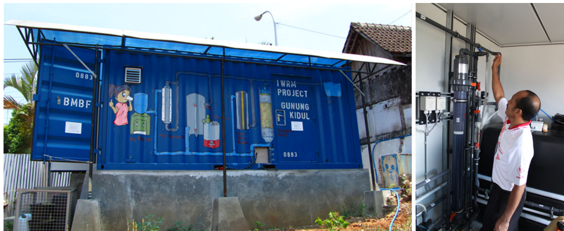
Fig. 7 Field laboratory installed at hospital of Wonosari. Left Picture explains the water treatment technologies in Indonesian language, as the laboratory is situated next to the future public parking for the hospital. Right Inside container
