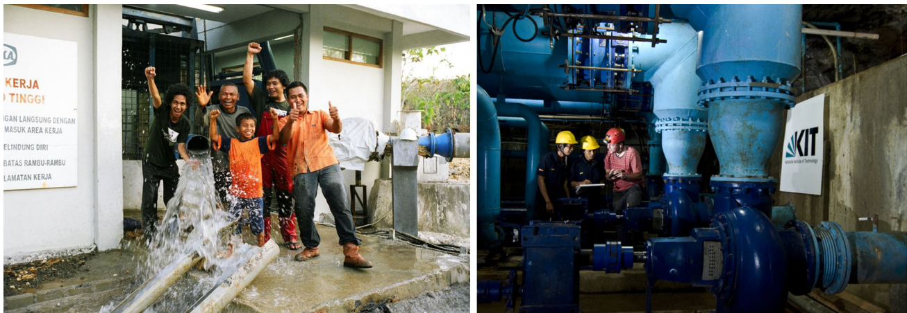
Fig. 16 Accomplishment of the first operational test ( left ) and know-how transfer during the initial operational phase ( right )
