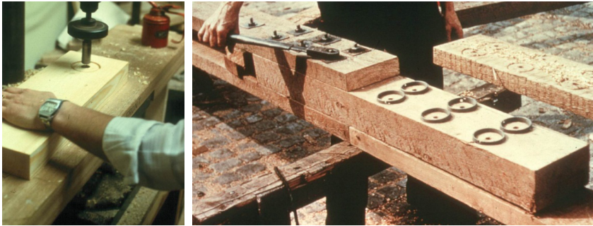
Figure E6-2 Left: Drilling the bolt hole and milling the depression for the connector. Right: Assembly of a joint with split ring connectors. (STEP 1995 Article C9)
