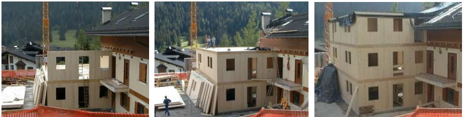
Figure B6-13 Construction progress of a CLT building; after 2, 4 and 6 days respectively. (Rasom S.r.l., Pozza di Fassa)
