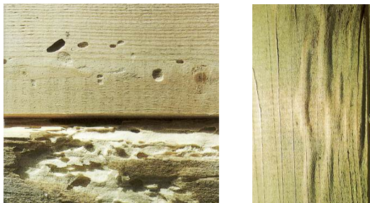
Figure B3-17 House longhorn beetle. Left: entrance holes and destruction under the intact wood surface. Right: Vein-like bulges, which point to the presence of a house long-horn beetle. (Sutter, 1997)
