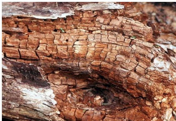
Figure B3-19 True dry rot with cubical cracks.
