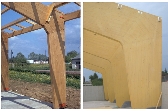
Figure E14-1 Examples for glued joints, frame corners with large finger joints and an interim piece. (photo on the left: H. Damm, photo on the right: H. Brünninghoff)
