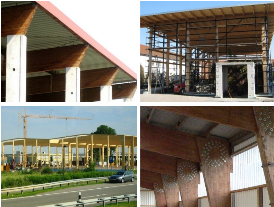
Figure G4-13 Circumstances, which may lead to damage. Error source planning/execution: torsional restraints at supports not built (top left), error source building physics: possible crack formation in glulam by local heating/drying behind planned glazing (top right), error source assembly: weathering of glulam (lower left) and construction of dowel circles, in which residual stresses are caused by shrinking (lower right).
