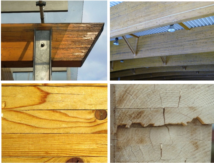
Figure G4-2 Initial damages – rot (top left), blue stain or mould fungi (top right), cracks in grain direction (minor shrinkage cracks, lower left), shear failure (part of beam in compression zone protruding at end grain, lower right).
