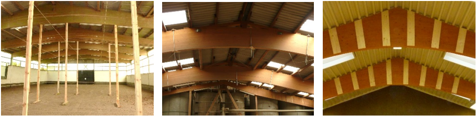
Figure G4-3 Cracks in pitched cambered beams, immediate propping/safeguarding required (left and centre), professionally retrofitted beams (right)
