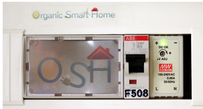
Figure 6.13: Raspberry Pi 3 Model B running the OSH in the ESHL at the KIT and the corresponding circuit breaker as well as the power supply (from left to right)
