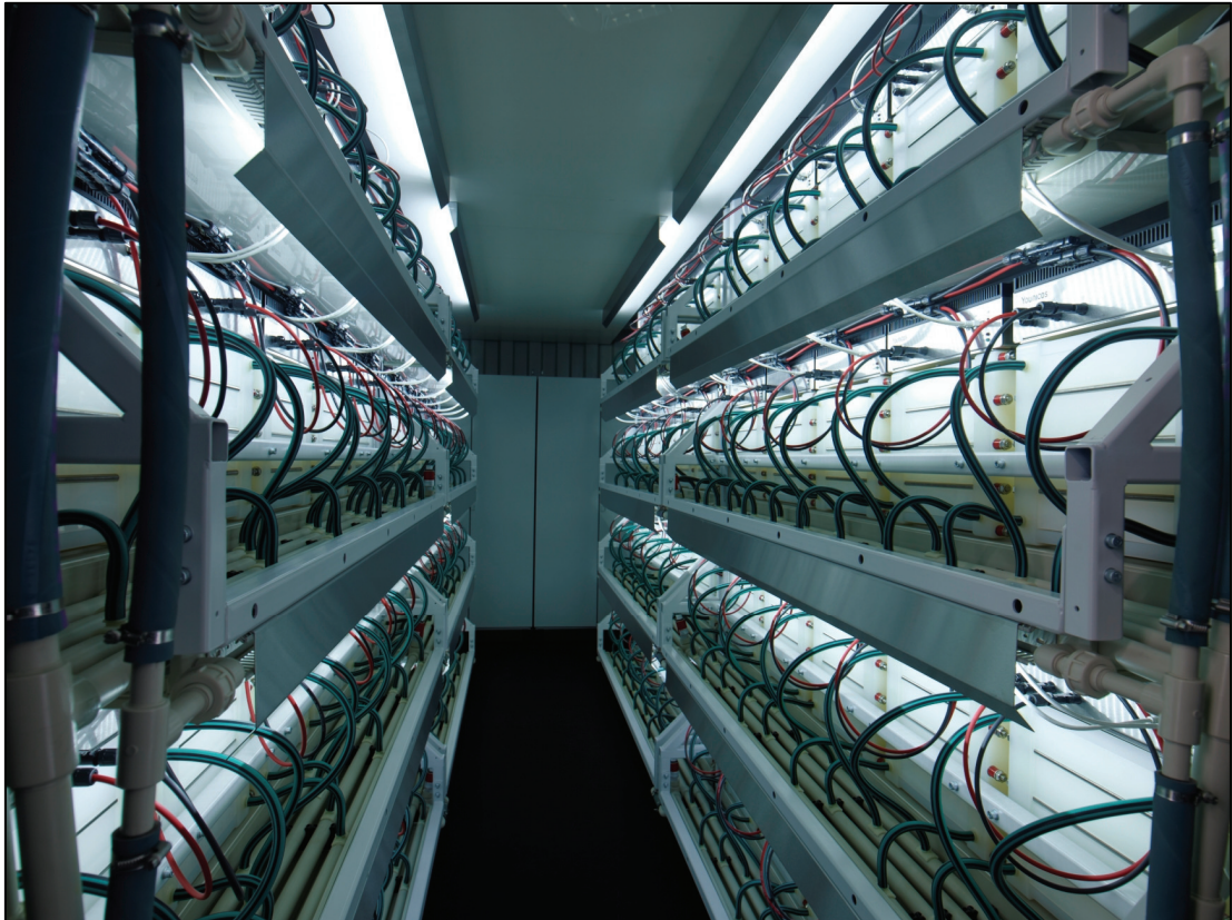
Figure 1-7: Interior view of a Gildemeister CellCube container; Copyright by Gildemeister Energy Storage GmbH, used with permission
