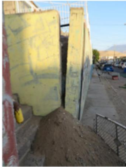
Fig. 1-4 Rotated retaining wall during the 2014 earthquake in Iquique, Chile, – Courtesy of G. Candia (Sitar, N., Wagner, N. 2015).
