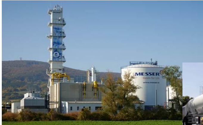
air separation unit (ASU)
