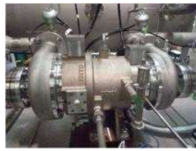
1st - 2nd Compressor
