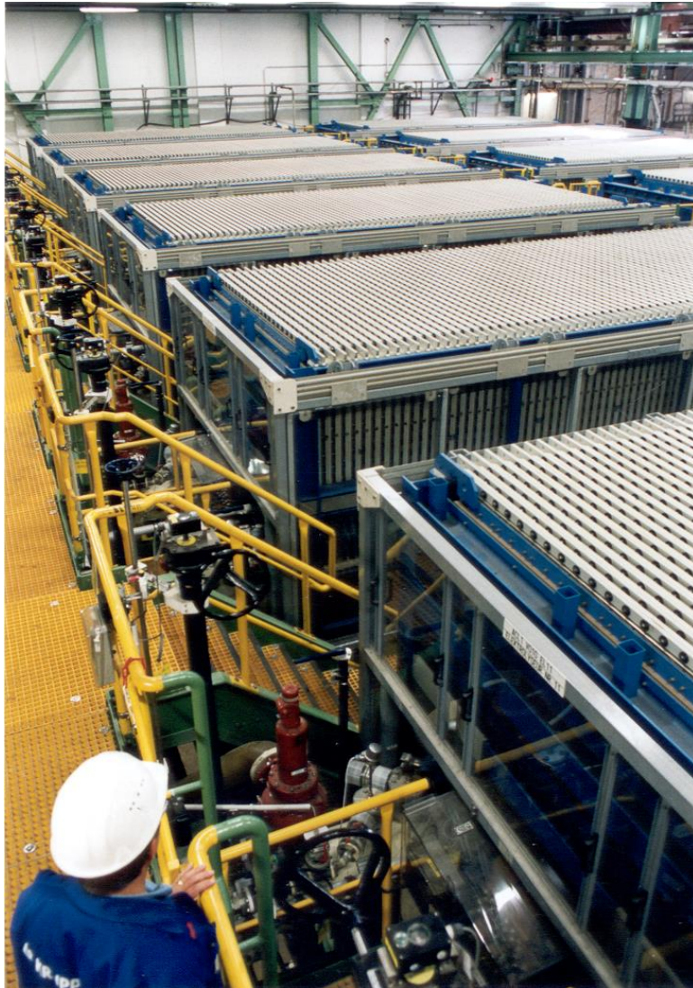
Chlorine elektrolysis, 20 kA
