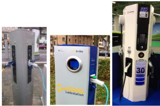
Figure 2: CROME interoperable public charging stations: 2 x “mode 3” (type 2 and 3) in Strasbourg (left), 2 x “mode 3” (type 2 and 3) in Kehl (middle), and 43 kW DC fast charging mode 4 in France (right).
