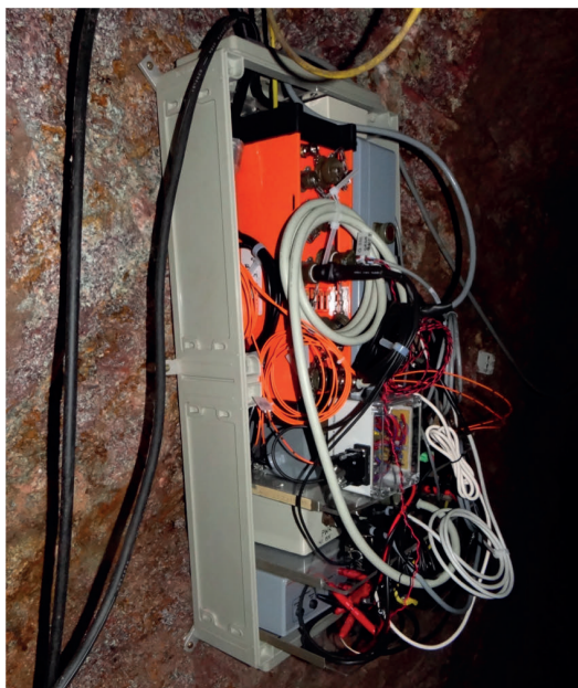
Figure 4.2: Electronics cabinet (with the cover removed) in the upper tunnel of the Anton mine. It houses the electronics units of the FGE and Overhauser magnetometers, the Q330 digitizer, the buffer amplifier, fiber optic media converters for LAN and PPS signals, a mini-PC, a Hygrometer and power supplies.
