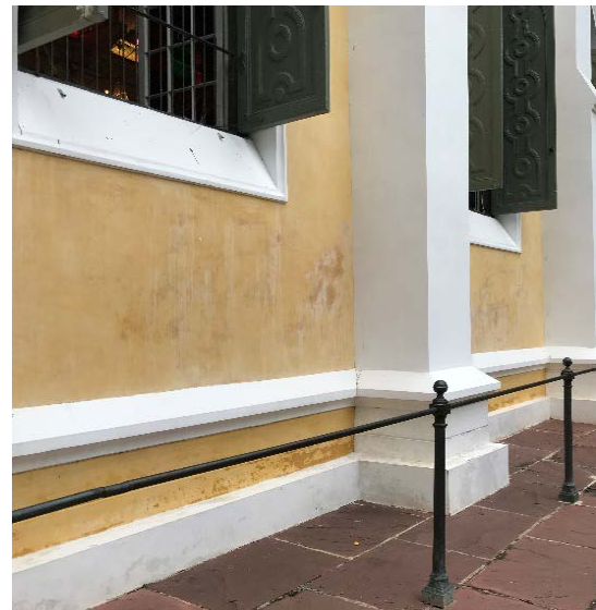
Figure 3: Signs of post-retrofit moisture problems.
