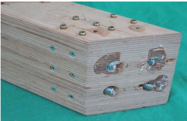
Figure 11: Failure of a tension diagonal with glued-in rods
