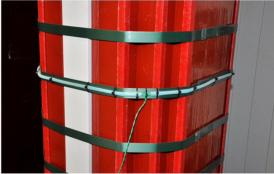
Figure 5.5: Pick-up coil around the limb of the transformer iron core. The coil is placed in the middle between the top and the bottom core yoke
