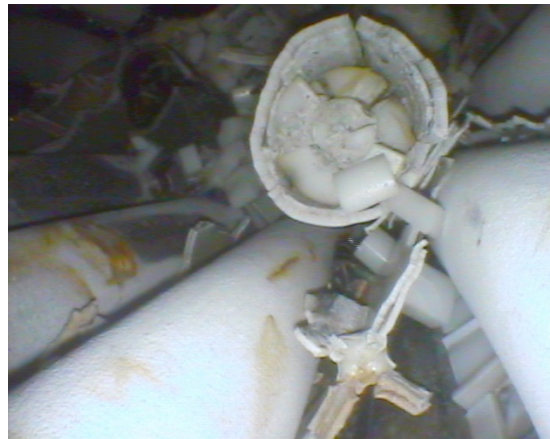
1120 mm: top of broken rod #5
