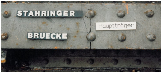
Figure 4.12: Stahringer bridge main girder - Crack after fatigue failure.
