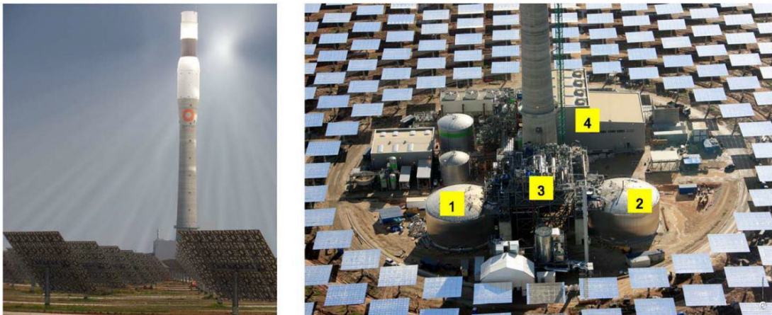
Figure 2.2: Pictures of Gemasolar, left: central receiver tower with heliostat mirrors in standby; right: (1) hot tank, (2) cold tank, (3) heat exchanger, (4) power block [21]
