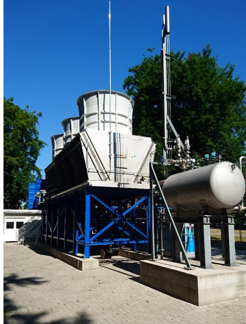
Fig. 8: Test facility MONIKA with a Rankine cycle of supercritical propane.
