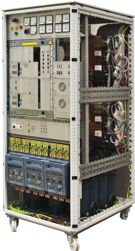
Fig. 7: Photography of the used inverter cabinet. It consists of an active-front-end inverter, two machine inverters and a real-time signal processing system.
