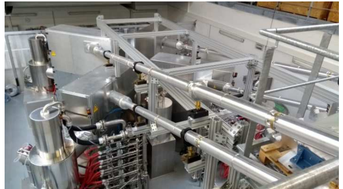
Fig. 1. Gyrotron installation ECRH3 at ASDEX Upgrade.
