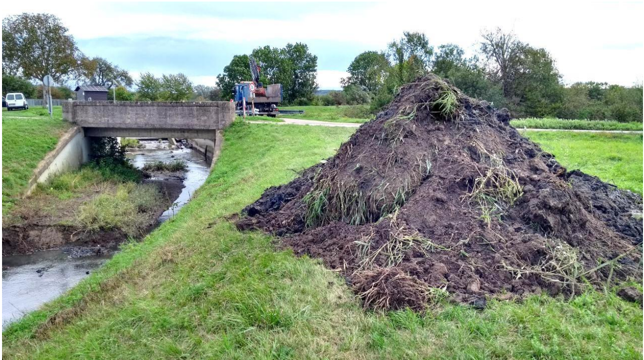
Figure 78: Top: Excavation of sediment deposited during and after the July/August high flow event 2019 in the Kraichbach/Kriegbach flood relief channel, ~7km downstream of the Ubstadt gauge. Bottom: Excavated material and yet to be removed in-channel deposits. Photo by the author, 1 st of Oct 2019.
