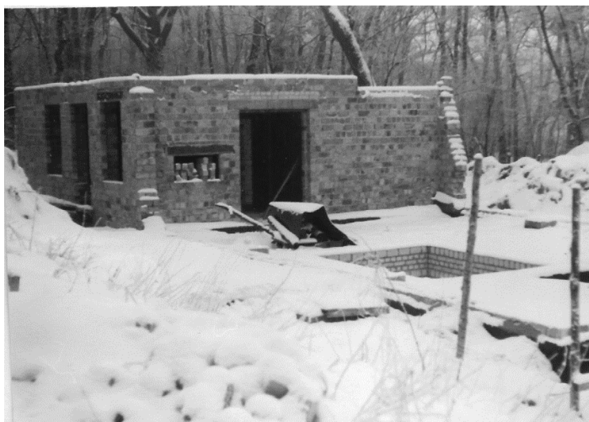
Figure 2. Construction site of the first high pressure hall with a pit for the triaxial press (6 January 1971).
