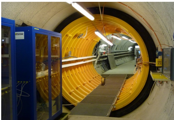
Fig. 1: The mega-packer system of the CFM experiment at the Grimsel Test Site. The shear zone is sealed with resin layer and surface packers are installed at outflow points on shear zone intersection. Pressurised water in annulus provides mechanical support to resin layer to counteract hydraulic head in the shear zone.
