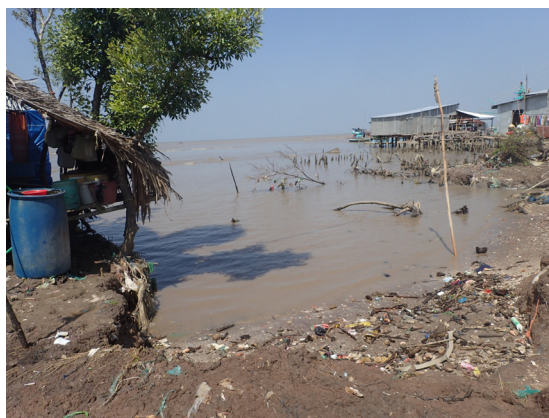
Fig. 1: Buildings in the Mekong-Delta endangered by coastal erosion (Image credit: Wendy Gonzalez Otero, KIT).
