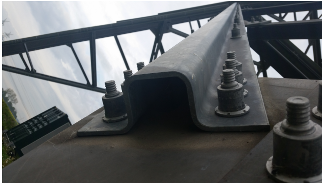
Figure 2.24: Lockbolts of the Butzkies tower and diagonal member with hat cross section. Photo: A. Struve 2018
