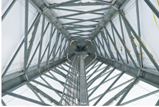
Figure 2.21: View into the pentagonal space frame lattice tower of GE [77]
