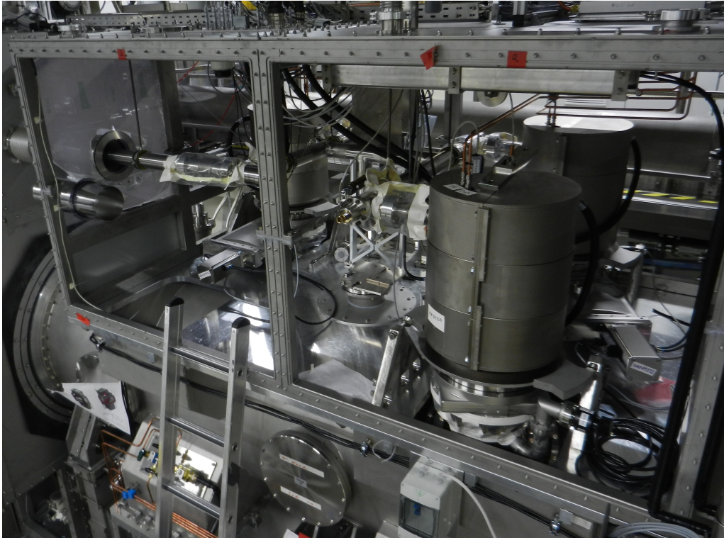
Figure 3.7.: DPS1-F top pumps and piping during commissioning. Shown are the top pumps and piping of the DPS1-F1 and DPS1-F2 pumping ports. The instrumentation on the bottom of DPS1-F1 and DPS1-F2 is similar. This setup is mostly mirrored by DPS1-R.
