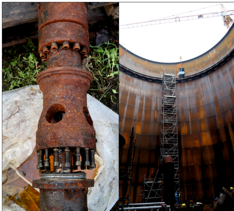
Fig. 4 Left: Corroded well pump of the cold well of the HT-ATES in Neubrandenburg. Right: New artificial storage tank to balance the short-term supply-demand mismatch (Fleuchaus et al. 2020a)
