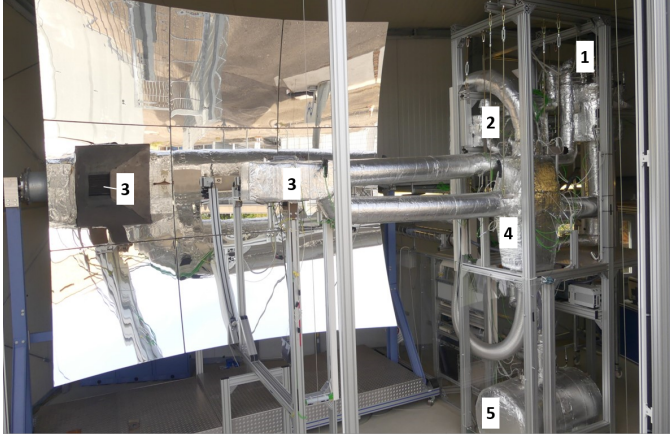
Figure 3: Picture of the SOMMER facility on-axis arrangement, taken by Mueller-Trefzer/KIT; 1: pump buffer tank, 2: heater, 3: receiver and copper shield (front and back), 4: cooler, 5: sump tank
