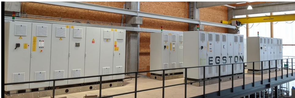
Figure 3.14: Five 200 kVA GAMP6 Egston switched-mode power amplifiers (1 MVA in total).
