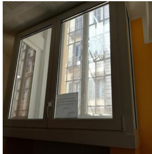
Figure 15. The new PVC window (on the front) and the original window (behind). Photo took on the ground-floor (the external window is shared with the mezzanine level). The sign asks to occupants to avoid operating the window due to the presence of mechanical ventilation.
