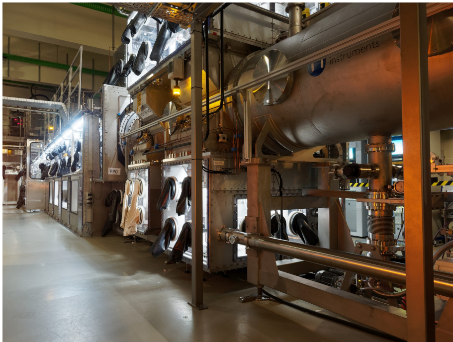
Figure 13. A View along the beam line. Shown on the right side is a part of the WGTS magnet cryostat with the glove boxes around the DPS1-F pumps (top and bottom). To the left follows the glovebox system around DPS and CPS .
