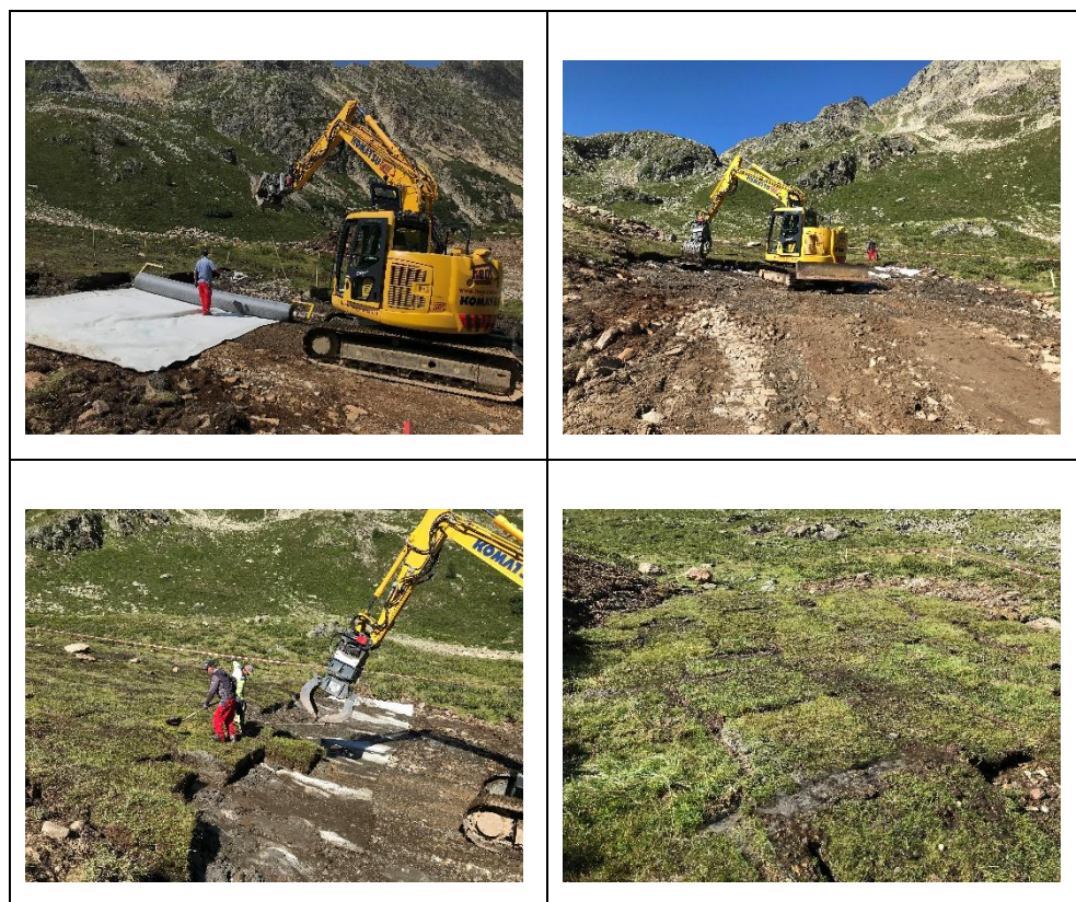
Fig. 3. Transplantation of an alpine Carex fen: Workflow at the receiving site. (a + b) preparation of the underground, (c) positioning of the turfs, (d) mosaic right after the transplantation
