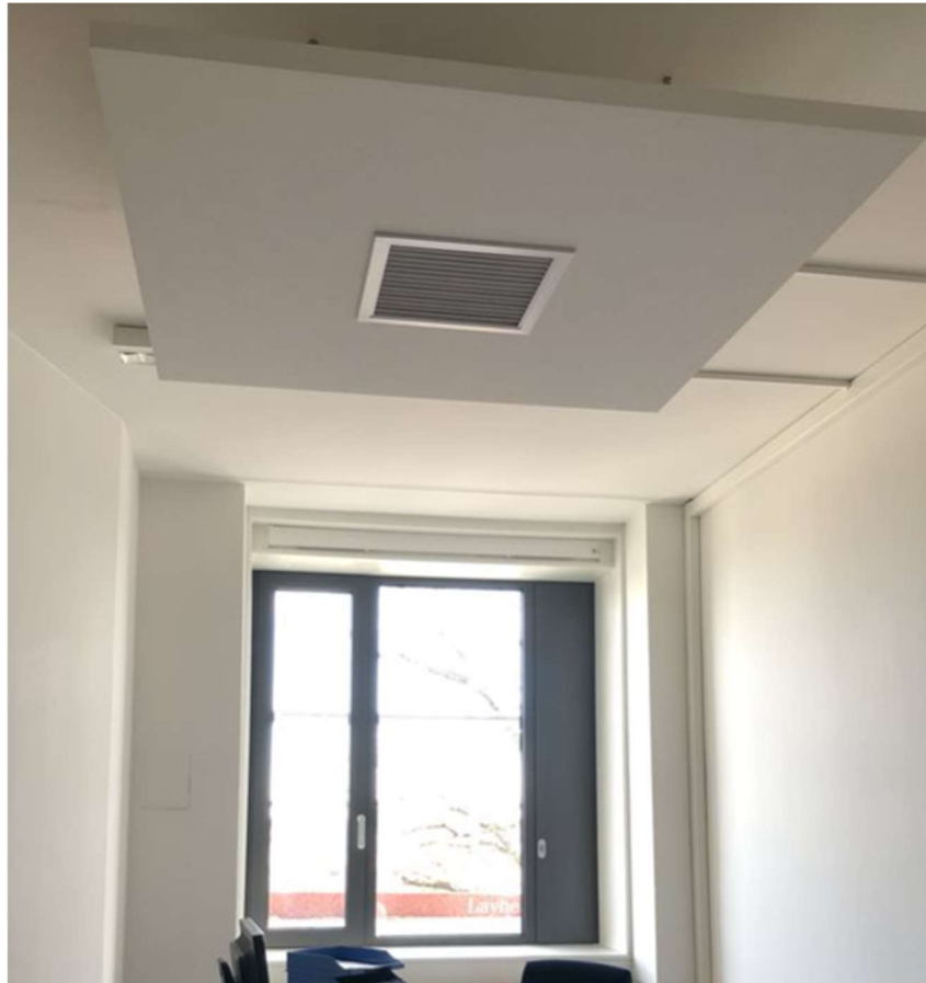
Figure 4: Inside view of an office room. The window system and the integrated personal ceiling fan are shown (Bergische Universität Wuppertal)
