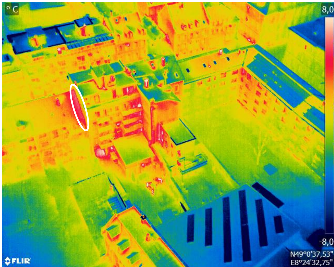
Figure A27. Example: thermal bridge of a connection between a rooftop and a wall.
