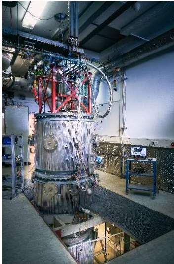
Figure 20: Research Entrained flow GASifier REGA
