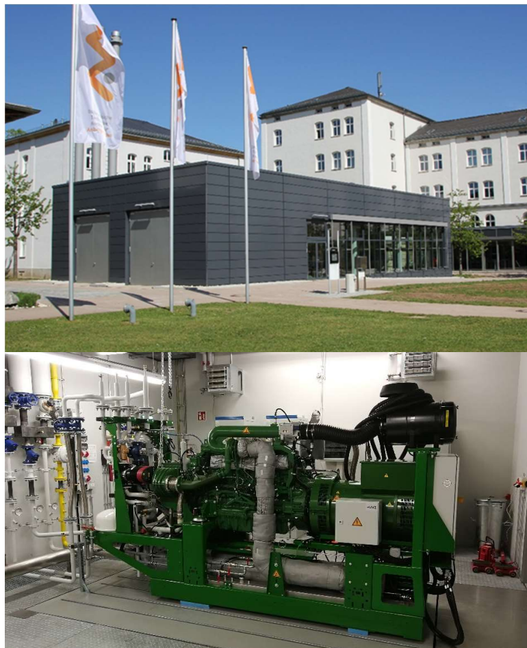
Figure 17: The CoECogen laboratory building in Amberg (top) with one of the test benches (bottom)
