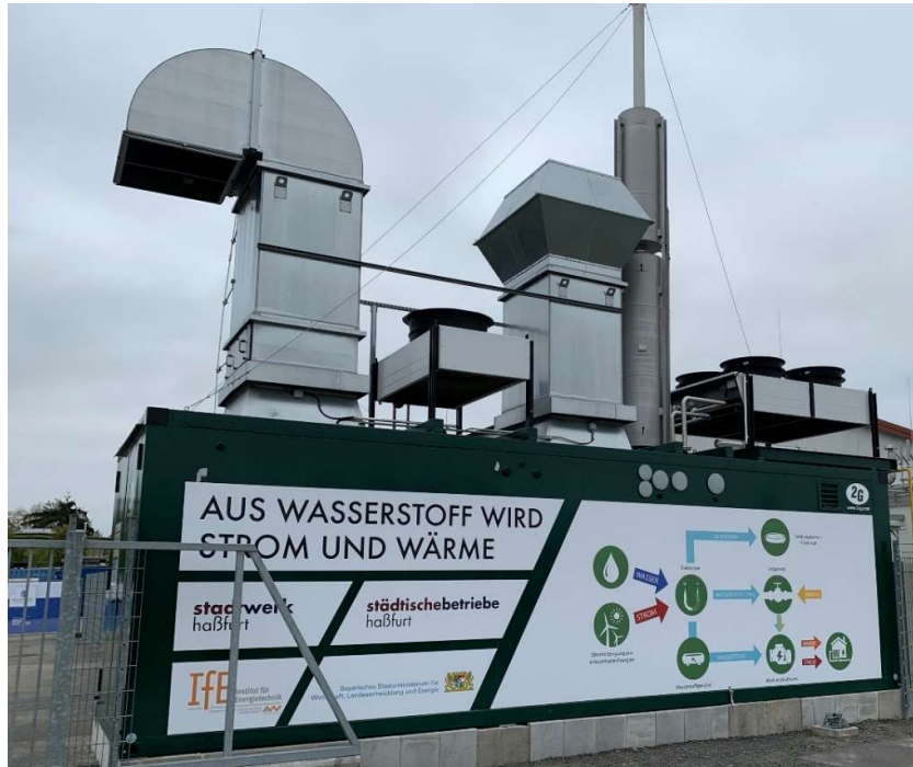
Figure 18 The hydrogen powered CHP unit in Haßfurt
