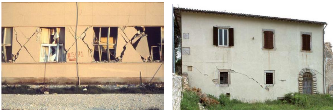
Figure 1.14: Diagonal shear cracking in brick masonry piers of a three-storey building (on the left), in stone-masonry piers of a historic building (on the right) after an earthquake [19]
