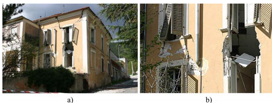
Figure 1.21: Flexural failure of spandrels in an old URM building after the earthquake on 6 April 2009 in L'Aquila (Italy): (a) Entire structure, (b) detail of a spandrel [30]
