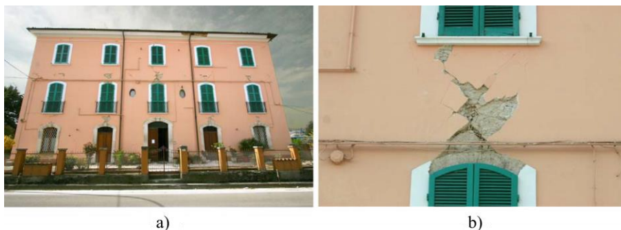
Figure 1.20: Shear failure of spandrels supported by shallow masonry arches in an old URM building after the earthquake on 6 April 2009 in L'Aquila (Italy): (a) Entire building, (b) detail of a spandrel [30]
