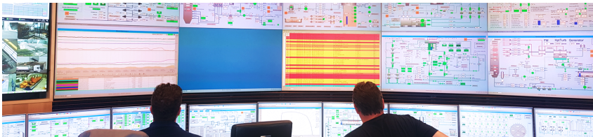
Figure 5.1: The control room at the Rheinhafen steam plant in Karlsruhe.
