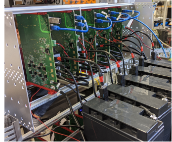
(b) A single phase of the converter viewed from the back, showing the lead-acid batteries
