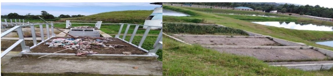
Figure 4.24: Screened non-biodegradable and biodegradable organic matter (left) and the drying beds (right) at the Bomet wastewater ponds system, Kenya
