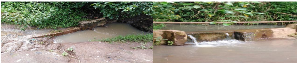
Figure 4.18: Lelechonik (left) and Ngomwet (right) Community Water Springs Rehabilitation and Protection in Nyangores WRUA, in MRB
