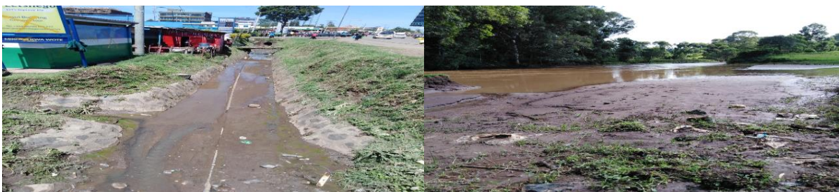
Figure 4.10: Drinking water main in the open sewer line, and visible solid waste and excessive siltation in Mara river, Bomet town, Kenya
