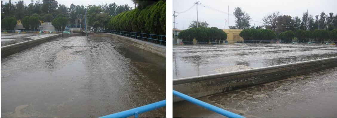
Fig. 1-7: Conventional activated sludge tanks from municipal WWTP Chapala, Mexico.
