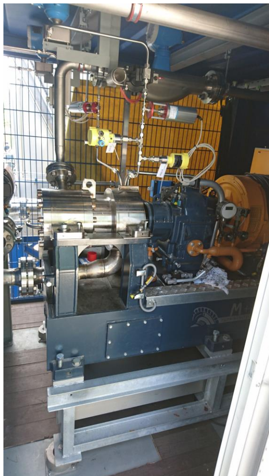
Fig. 5: Turbine with gearbox and generator
