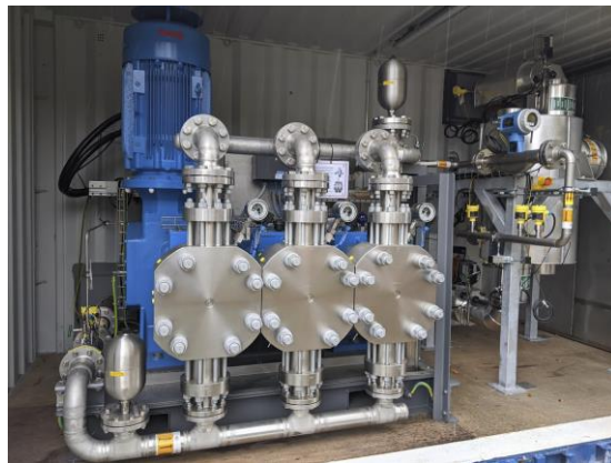
Fig. 4:Main pump and Plate heat exchanger
