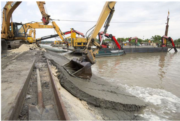
Fig. 3 Installation of a sealing clay layer under water condition (BAW Image archive)
