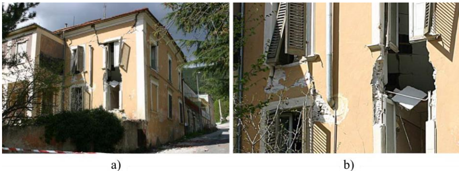
Figure 1.21: Flexural failure of spandrels in an old URM building after the earthquake on 6 April 2009 in L'Aquila (Italy): (a) Entire structure, (b) detail of a spandrel [30]
