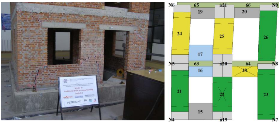
Figure 6.20: P2 wall of the BM model: experimental [73] and numerical final DLs (monotonic pushover in the +y direction with triangular inverse load pattern)
