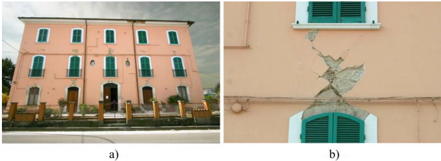
Figure 1.20: Shear failure of spandrels supported by shallow masonry arches in an old URM building after the earthquake on 6 April 2009 in L'Aquila (Italy): (a) Entire building, (b) detail of a spandrel [30]
