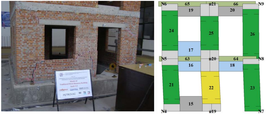
Figure 8.1: P2 wall of the BM model: experimental [73] and numerical final DLs (monotonic pushover analysis in the -y direction with load pattern proportional to the masses)
