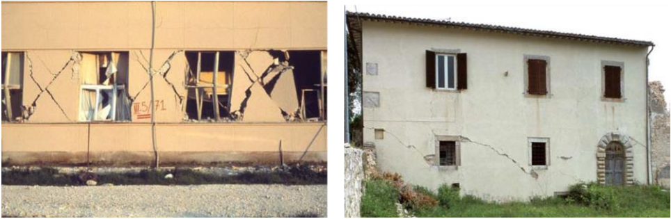
Figure 1.14: Diagonal shear cracking in brick masonry piers of a three-storey building (on the left), in stone-masonry piers of a historic building (on the right) after an earthquake [19]
