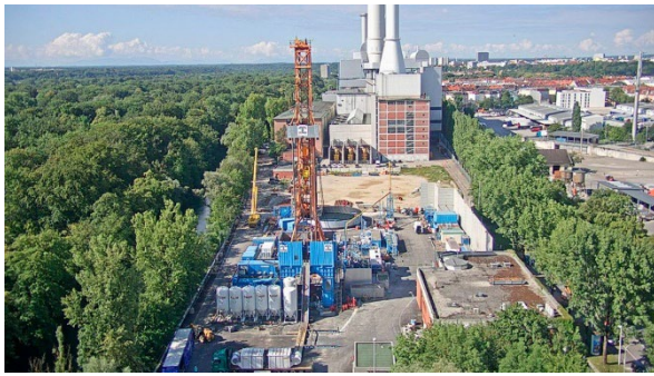
Figure 3: Renewable heat generation: Construction site of Germany's largest geothermal plant in Munich (Schäftlarnstrasse)
