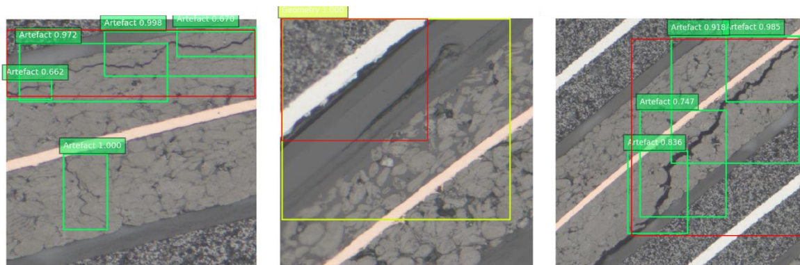
Figure 4-15: Examples where the Faster R-CNN model with ResNet-50 feature extractor correctly detected the defect but incorrectly predicted the bounding box coordinates. For instance, the model assigned several bounding boxes (green box) to the same defect in the first image, while in the second image, the assigned bounding box is much larger than the ground truth (red box). This would affect the total number of defects reported by the system.
