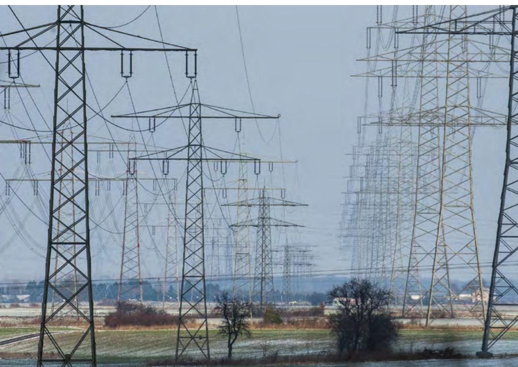
Environmentally compatible, efficient, flexible, and stable energy systems have to be customized for future energy supply.
