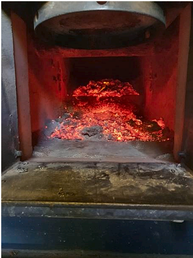
Fig. 15. Fuel bed of investigated grate furnace.
