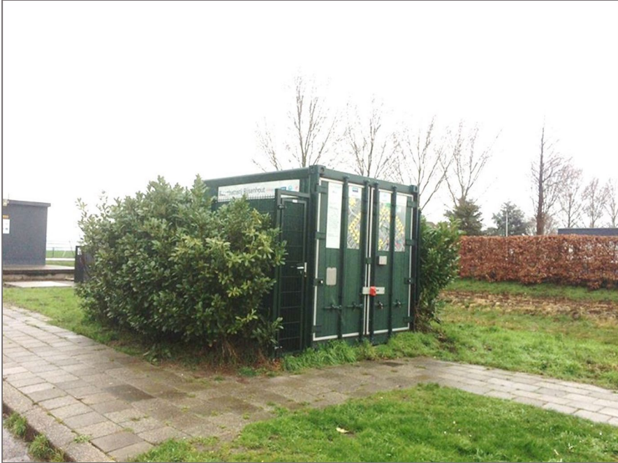
Fig. 3 The external appearance of the community battery. Source: Author
